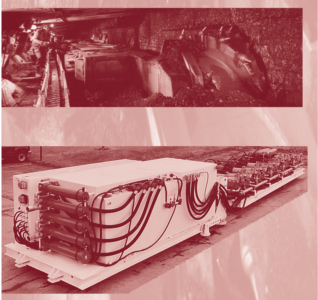
Water Service Filters in use.
