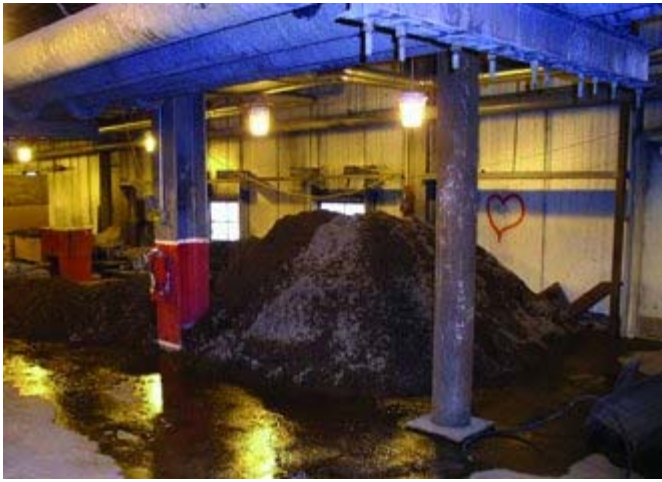
4. Ready for pickup. Piles of calcium carbonate scoured from North Omaha Power Station's five condensers await removal. Courtesy: Conco Systems Inc.
